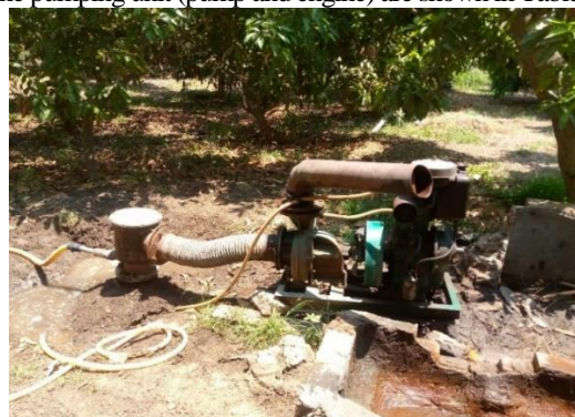
Fig. 4. Engine and pumping unit
