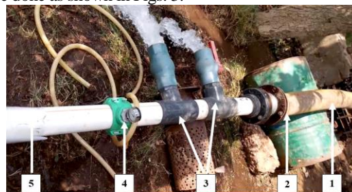
(1) From pump delivery (2) Flange 6 inch (3) Two valve 6 inch connected by T 6 inch (4) Pressure gauge (5) To Perforated Tube
